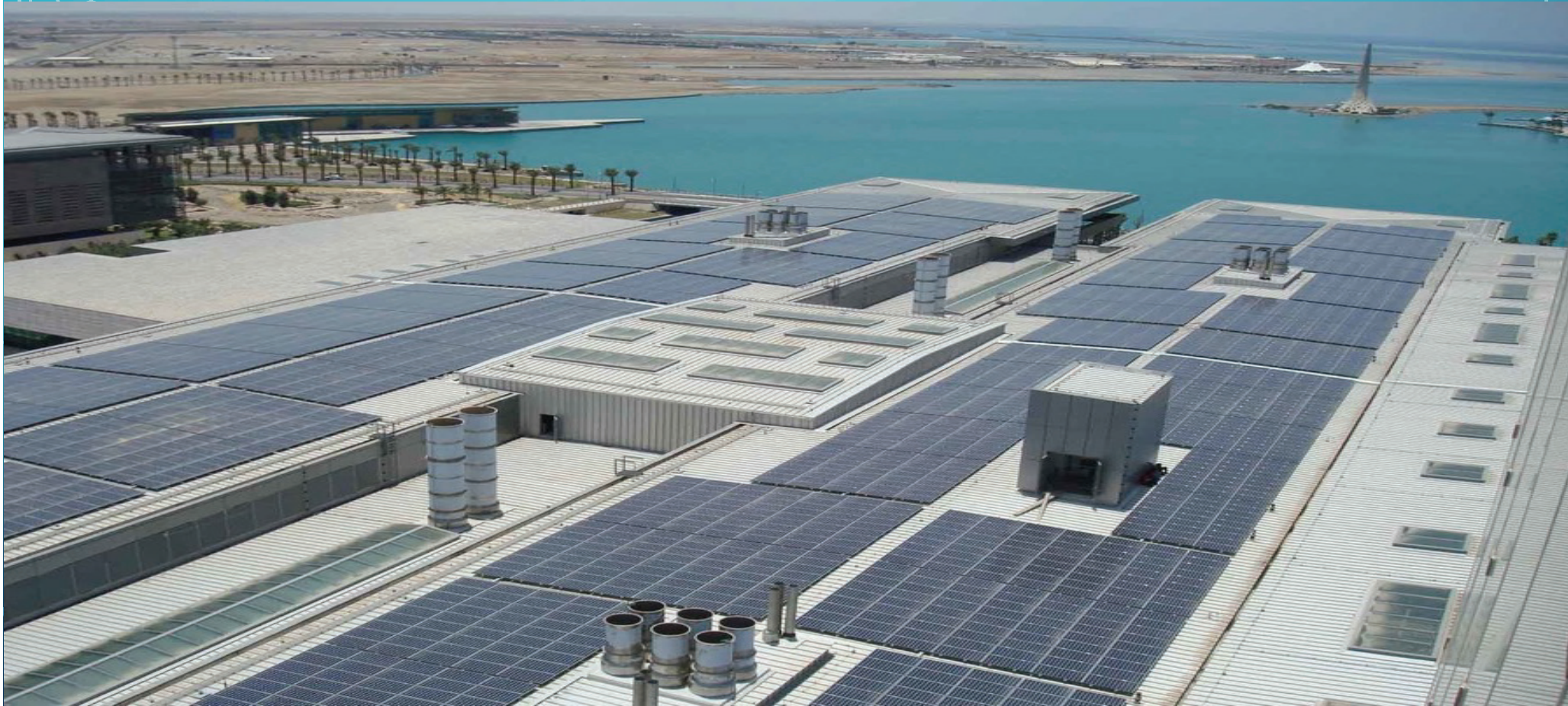
2-MW Roof-top Solar PV plant at KAUST
