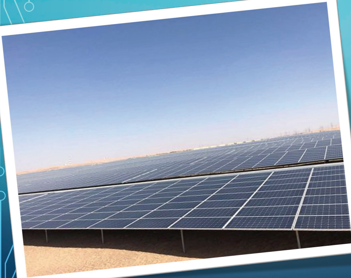
Solar PV Project in UAE
