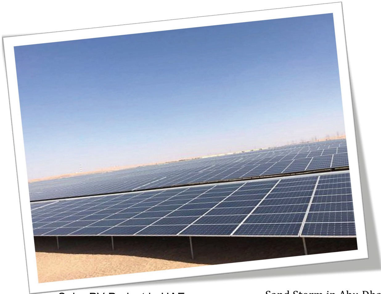
Solar PV Project in UAE
