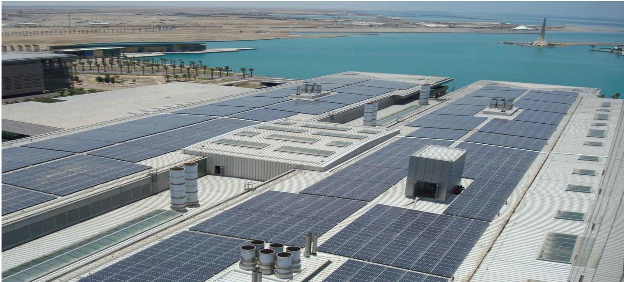
2-MW Roof-top Solar PV plant at KAUST
