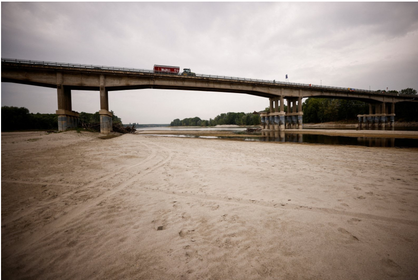
The Jialing Riverbed at the confluence with the Yangtze River is exposed due to drought on August 18, 2022 in Chongqing, China .
