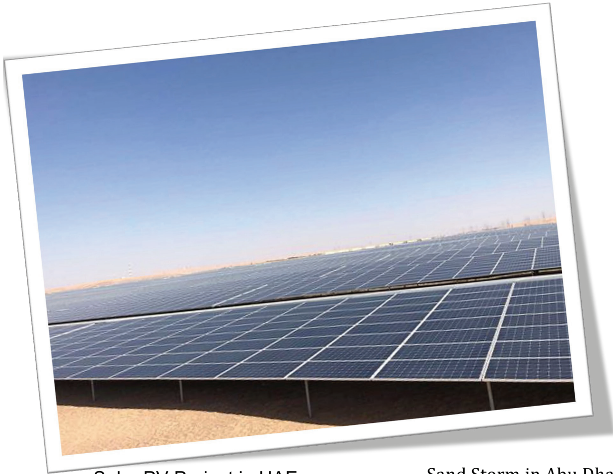
Solar PV Project in UAE
