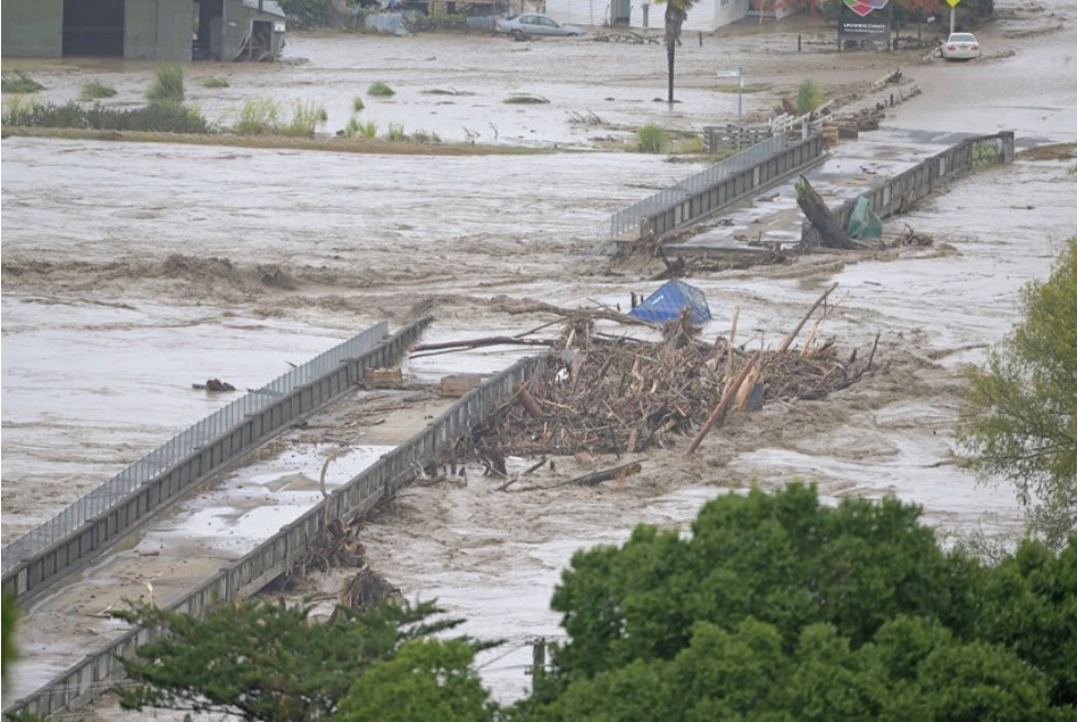
Aljazeera News, The Waiohiki Bridge is washed away in Napier. [Kerry Marshall/Getty Images]
